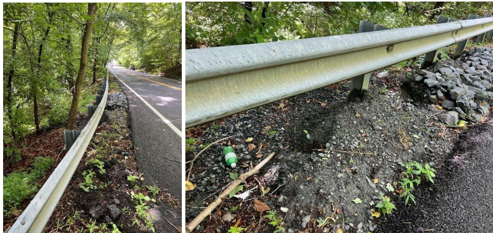
After repair: The side slope is already eroded by bad drainage (June 27, 2024)
