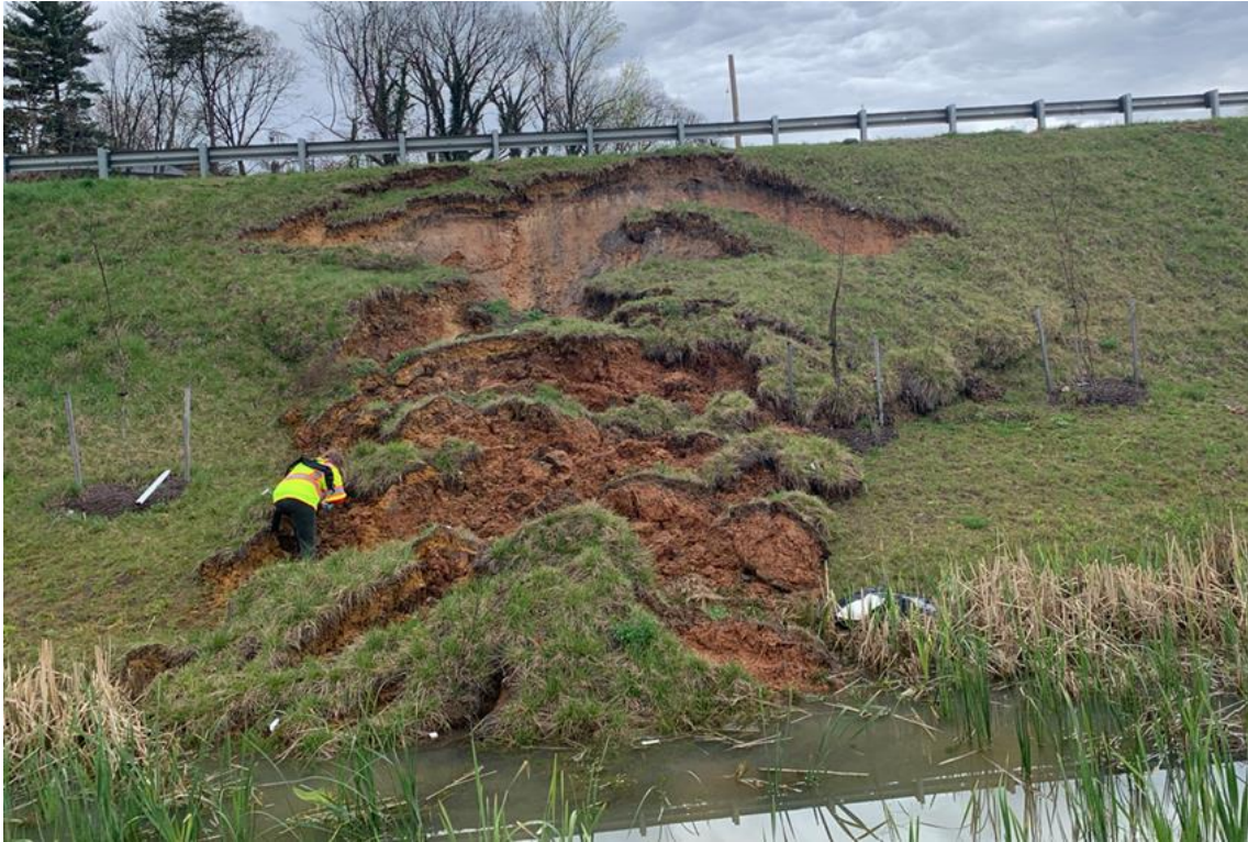
Figure 3.19. Landslide happened on April 4, 2024, at site 11.
