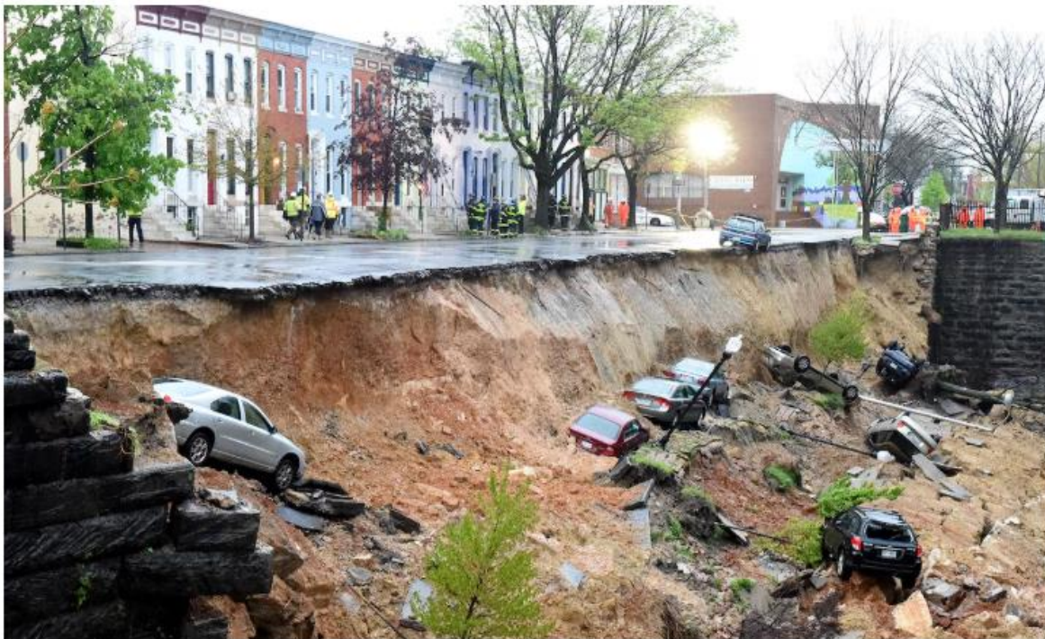
Figure 2.1: Retaining Wall failure leading to a Collapsed One Lane of East 26 th Street in Baltimore after heavy rain on April 30, 2014. (Berlin, 2014 nationalgeographic.com ; washingtonpost.com ).
