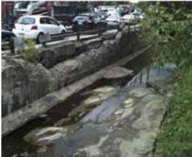
Saw Mill Run Creek Condition
