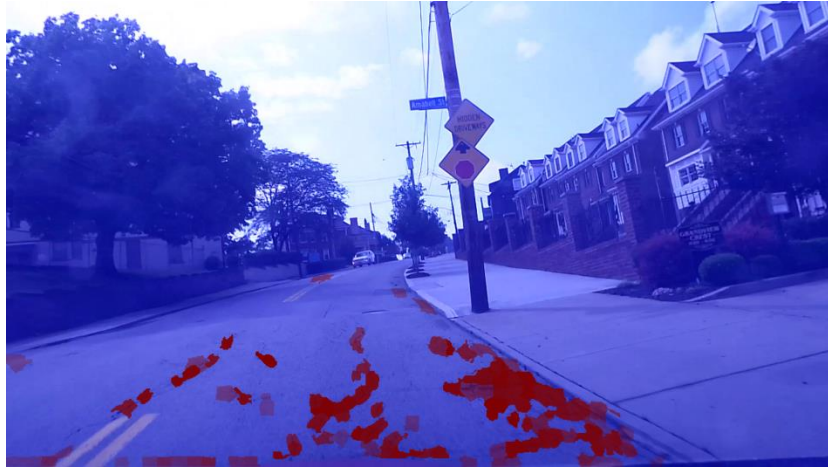
Figure 10 Classification result. The color indicates the severity of distress: blue = no cracks, red = cracks.
